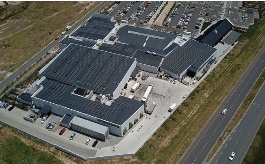
Solar panels installed on the roof of the Sitari Village Centre Mall, Cape Town, Western Cape province.
